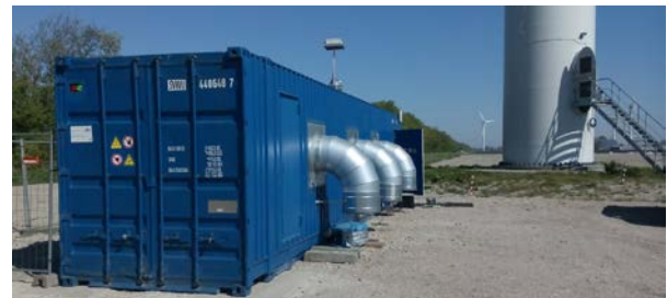
Figure 3: Test device installed close to a multi megawatt wind turbine.
