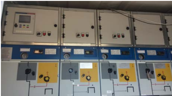
Figure 5: A 30 kV medium voltage switch gear including a grid protection relays.
